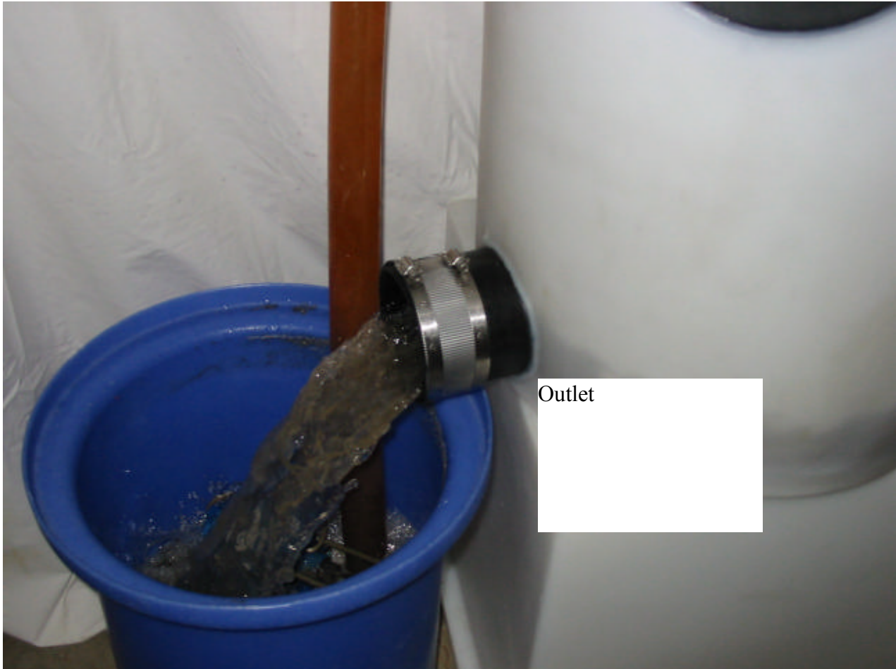
Figure 2. Example of treated water re-entering tank.
